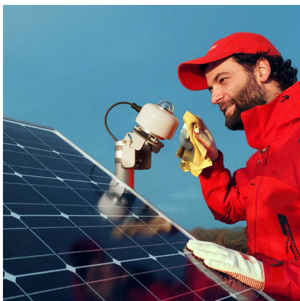
Figure 2 SR15-A1 pyranometer mounted in POA (Plane Of Array) on a mast for PV performance monitoring
