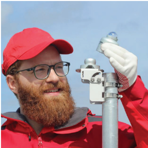
Figure 4 with PMF01, besides Plane of Array (tilted) installations, pyranometers can be mounted horizontally too, either on a crossarm, vertical mast, or on a platform. The photos show the installation of SR15 on a horizontal crossarm, and SR05, with its ball levelling mount, on a vertical mast. A spring-loaded bolt and tube clamps come included with PMF01.
